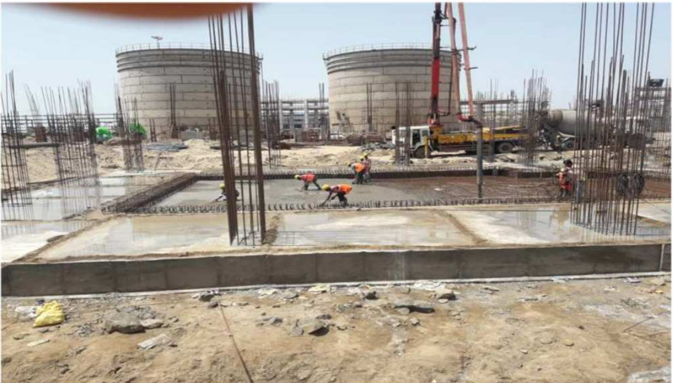
FIRE WATER TANK CONSTRUCTED AND WARE-HOUSE FOUNDATION IN PROGRES - LPG TERMINAL MUNDRA
